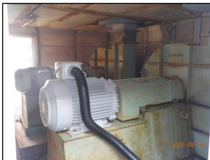
scrubber exhaust fans
