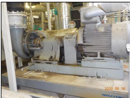
cooling water pumps for absorption refrigerators
