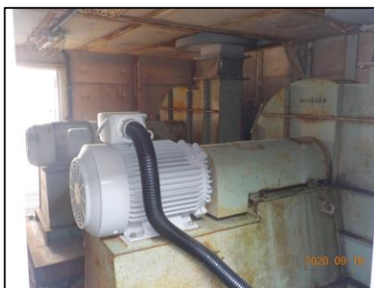
scrubber exhaust fans
