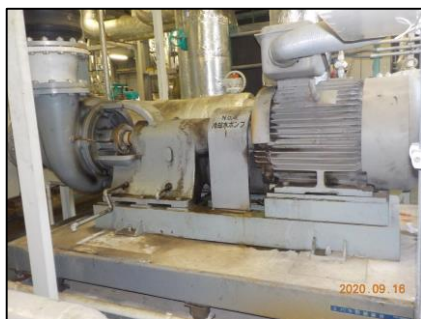
cooling water pumps for absorption refrigerators
